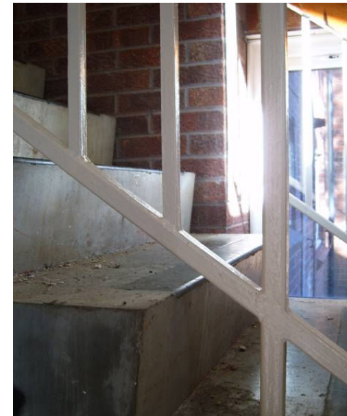
Photograph 2 – dirty stairs in Exhall Close
